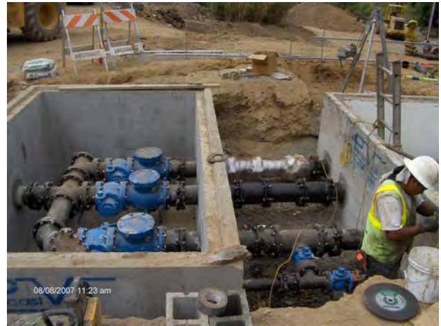
Stonecrest Lift Station
