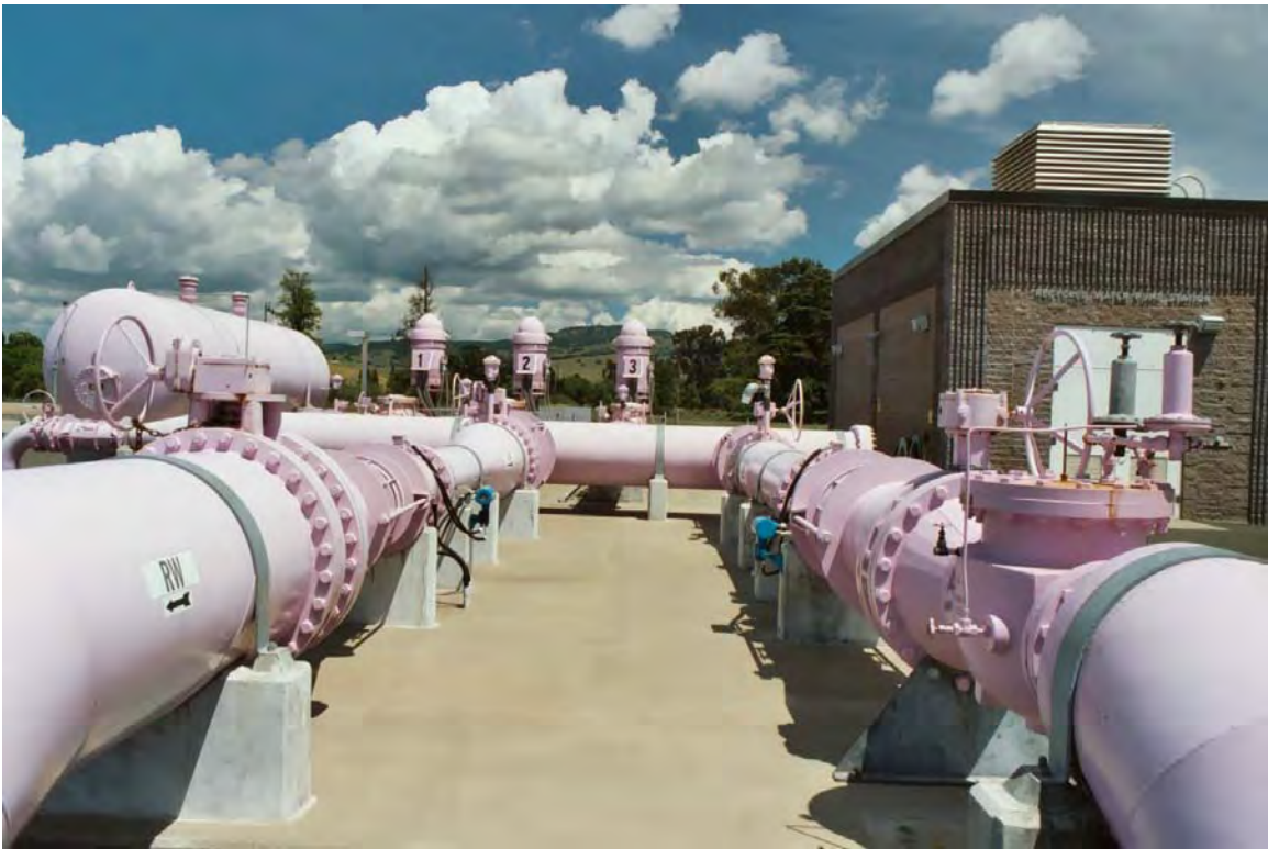
Recycled Water Pump Station – Soscol Water Recycling Facility
