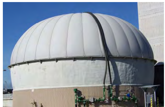
The Dystor cover is scheduled for replacement in FY 2015/16.
