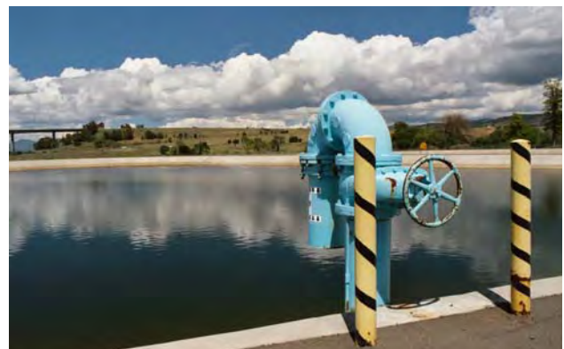
Recycled water storage
