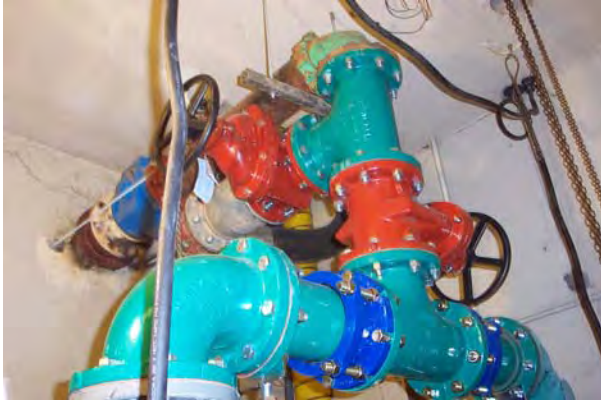
Valves at Riverpark Lift Station
