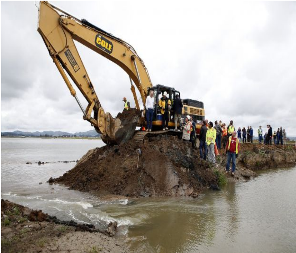
Photo 3a. A backhoe breaches the levee on April 25 at the Hamilton Wetlands Restoration Project (photo taken from SF Chronicle).
