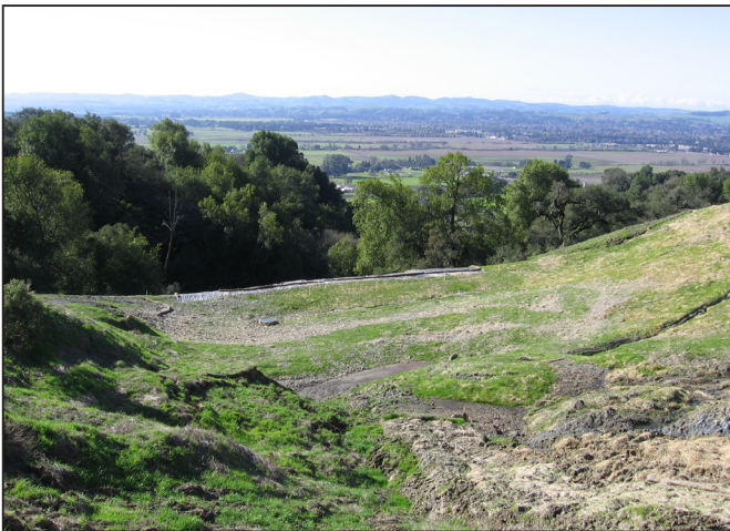
Photo c. Active slide face graded, drain pipes used to dewater surface drainage away from slide; drain, manhole cover, and detention area seen in mid-ground (Feb. 2006).
