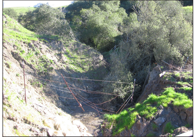
Photo b. Toe of active slide pushes eroded material directly into creek (Feb. 2006).
