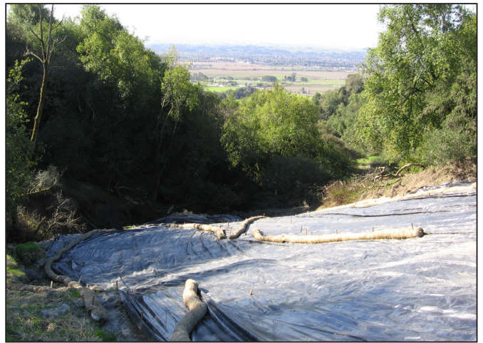
Photo d. Active lower slide face transports sediment directly to Cook Creek, this is below the area shown in Photo (c), plastics and wattles used to reduce slide saturation and erosion (Feb. 2006).
