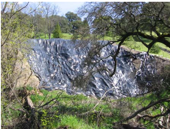
Direct view of slide face from vicinity of creek bank area below slide.
