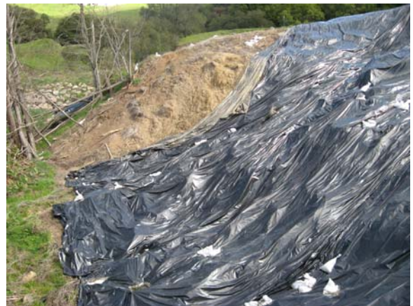
View of slide zone showing arcuate slide face in profile. Project treatments would include grading of slide face and strengthening toe of slide area with earthwork and tree plantings.
