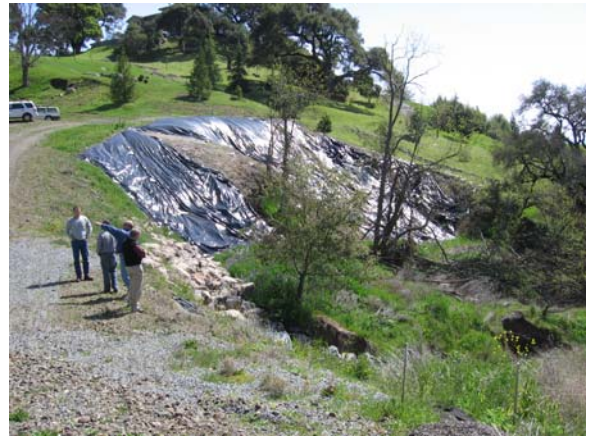
Nearer view of slide area showing head scarp adjacent to road, slide face, and base of slide in upland zone above creek.
