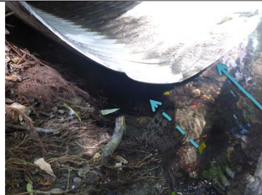
Photograph 4: Entrance of the culvert. The bottom of the channel upstream of the culvert was approximately three inches above the bottom of the culvert.
