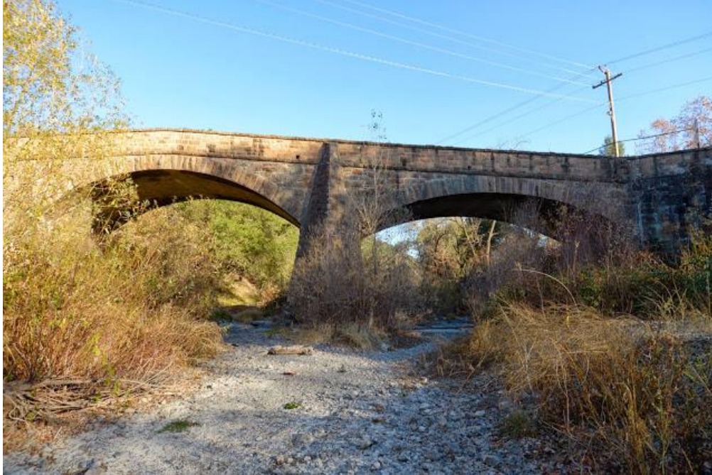
Dry Napa River at Pope Street Bridge (2013), Napa County, California Photo (unedited) by Mark Yashinsky (available at: http://bit.ly/2mBRET9 )
