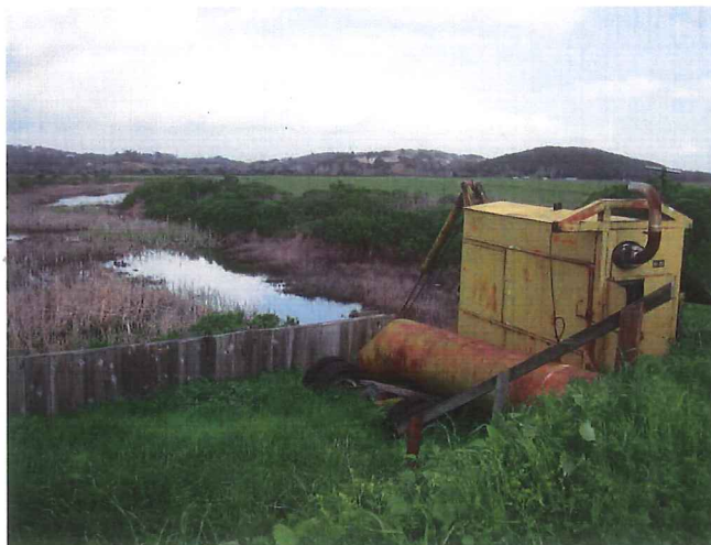
Big Bertha pump station at Simmons Slough.
