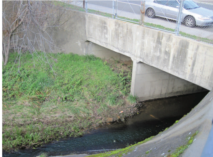
Arroyo de San Jose just upstream of Ignacio Blvd road crossing, showing area of sediment removal.
