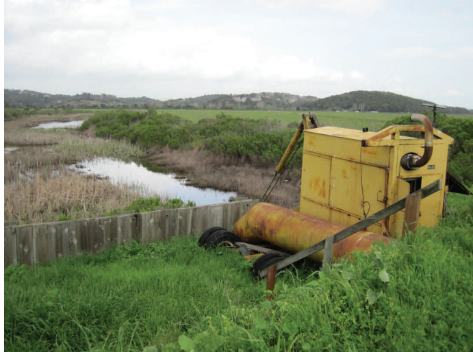
Big Bertha pump station at Simmons Slough.
