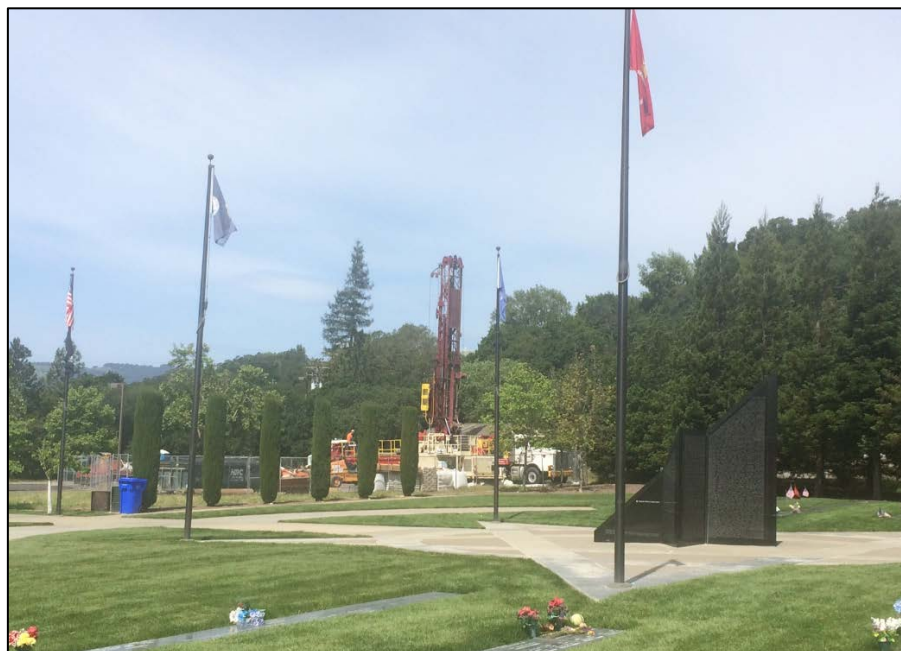
Figure 7. Photo showing location of ASR project near Veterans Memorial Park, with drill rig installing the ASR Well (TW6A) in the background.
