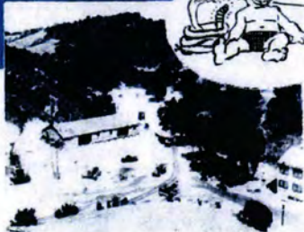
June 30, 1939, 11 days after ground-breaking, Permanente looked like this. Silos now stand in left foreground. Below, first thickener tank in skeleton stage.
