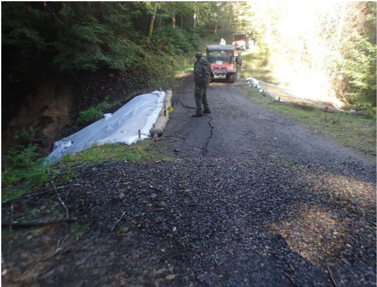
Figure 3. Cracking of Dark Gulch road prism around upstream sinkhole. The sinkhole has been covered with plastic tarp.
