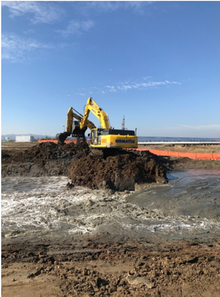
Photo 1. Suisun Bay enters the Project site as two excavators breach the levee.
