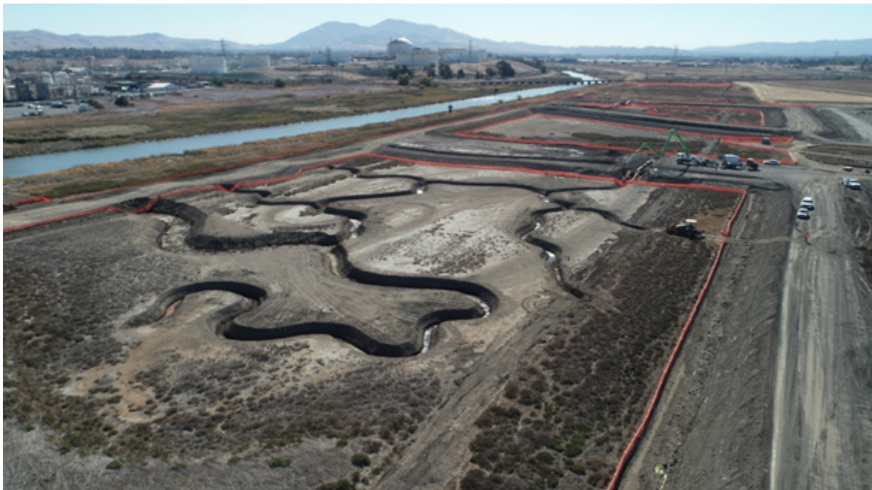
Photo 2. Newly excavated tidal channel network waiting to be connected to Walnut Creek. About six miles of orange fencing was installed and inspected and maintained daily to protect and exclude salt marsh harvest mouse from the Project construction areas.
