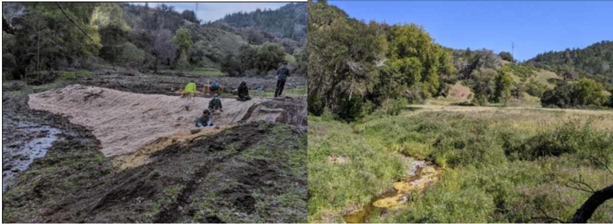
During construction (left) and after (right) photos of a post-fire emergency response installation of an erosion control blanket and willow sprigging within Sugarloaf Regional Park in Sonoma County.
