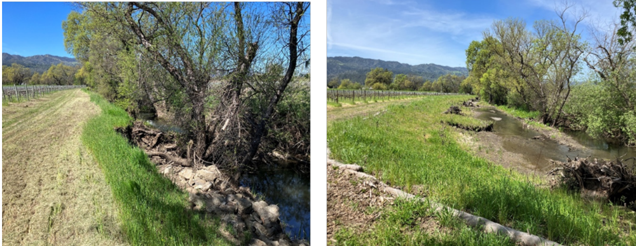
Figure 2: Group A - Site 5 of Bale Slough Bear Creek Restoration Project showing steep eroding banks before project implementation in April 2023 (left photo), and the same site with laid-back banks and large wood following construction in March 2024 (right photo).
