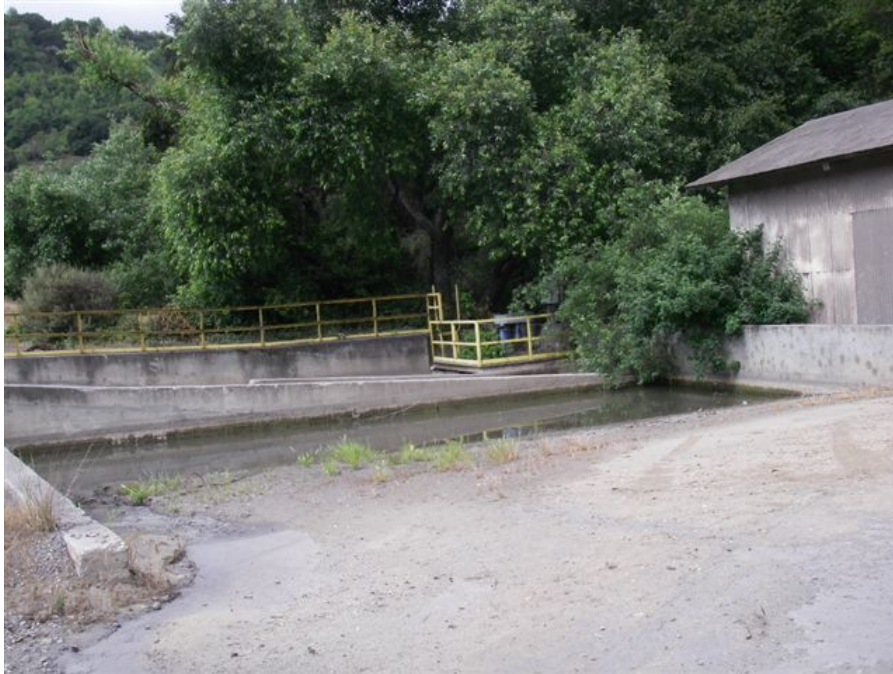
Photograph 11: Dinky Shed Basin. Note pump located just beyond the sump near the yellow railing
