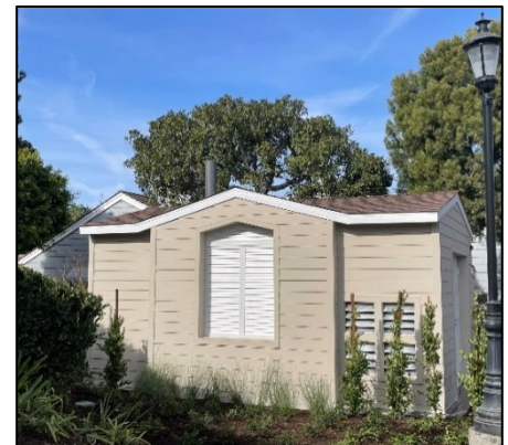
Above: Photo of the SVE System installed at Belcourt Terrace.
