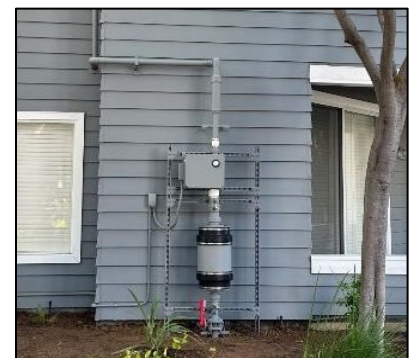
Above: Photo of an SSD System installed at Bayridge Park.
