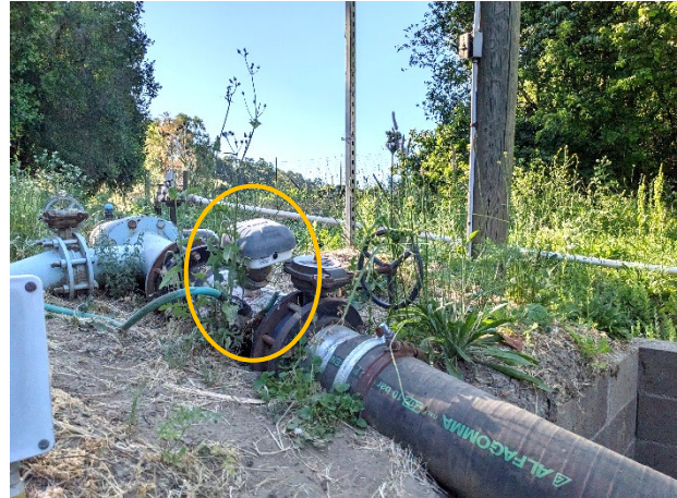
Figure 1. Pipeline for diverted surface water. An in-line water sensor and data logger are circled in orange.
