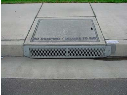
Catch Basin Screens
