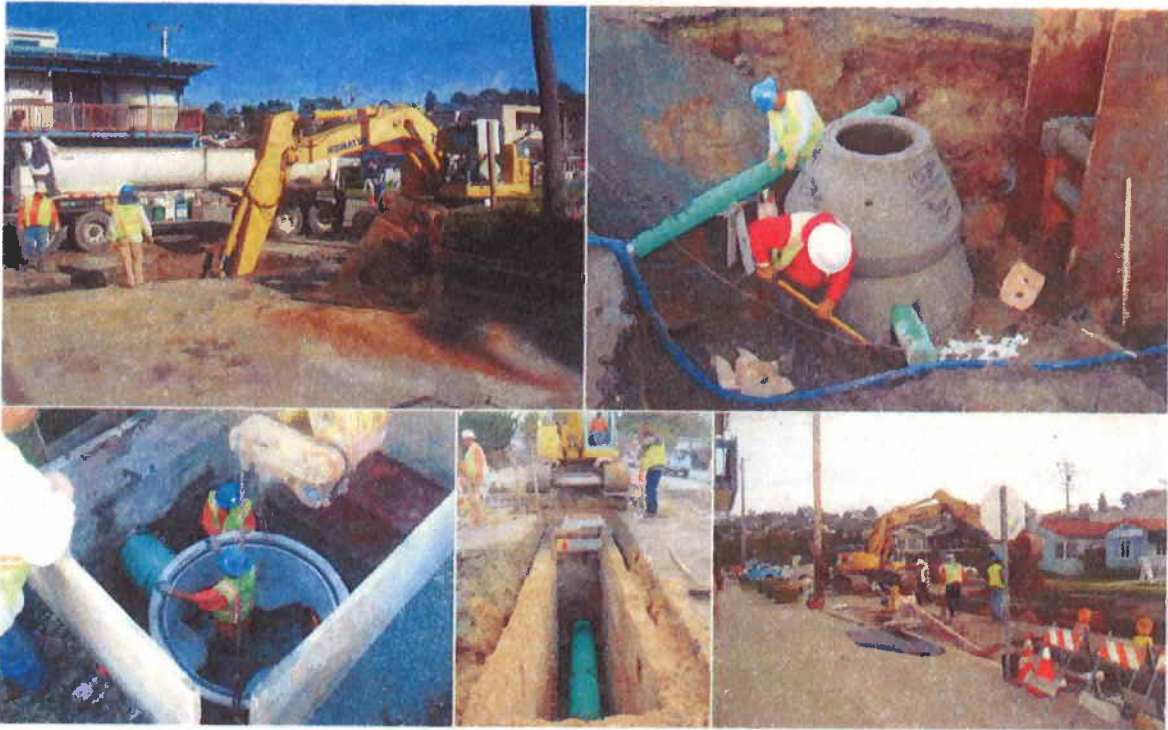
Top Left: Digging trenches for new transmission line. Top Right: Installing manholes. Bottom Left: Installing pipe. Bottom Middle: Installing pipe. Bottom Right: Construction site.
