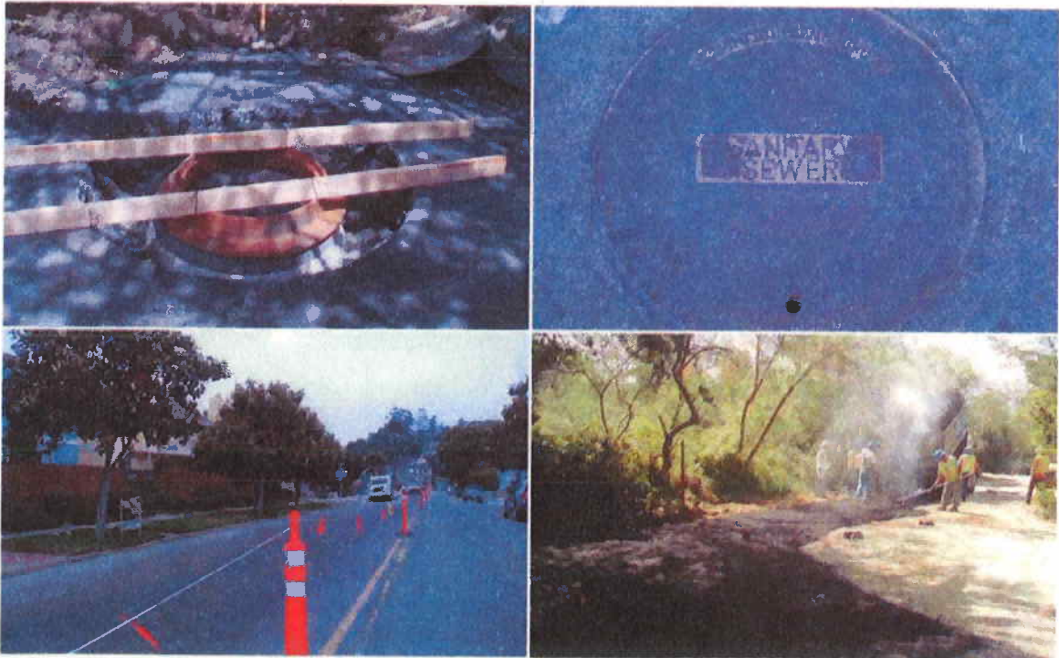
Top Left: Installing manhole covers. Top Right: Installed manhole covers. Bottom Left: Construction site after repaving. Bottom Right: Repaving construction site.
