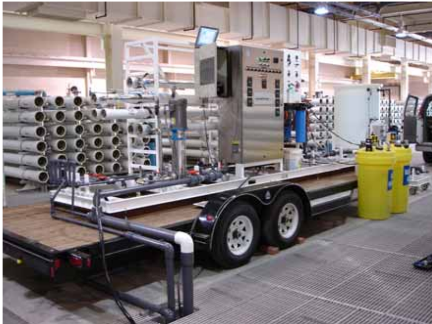
Figure 2.3. Pilot-scale membrane skid operational at a full-scale RO facility.
