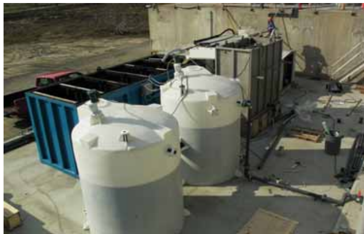
Figure 2.4. Pilot-scale MBR at Facility 1.
