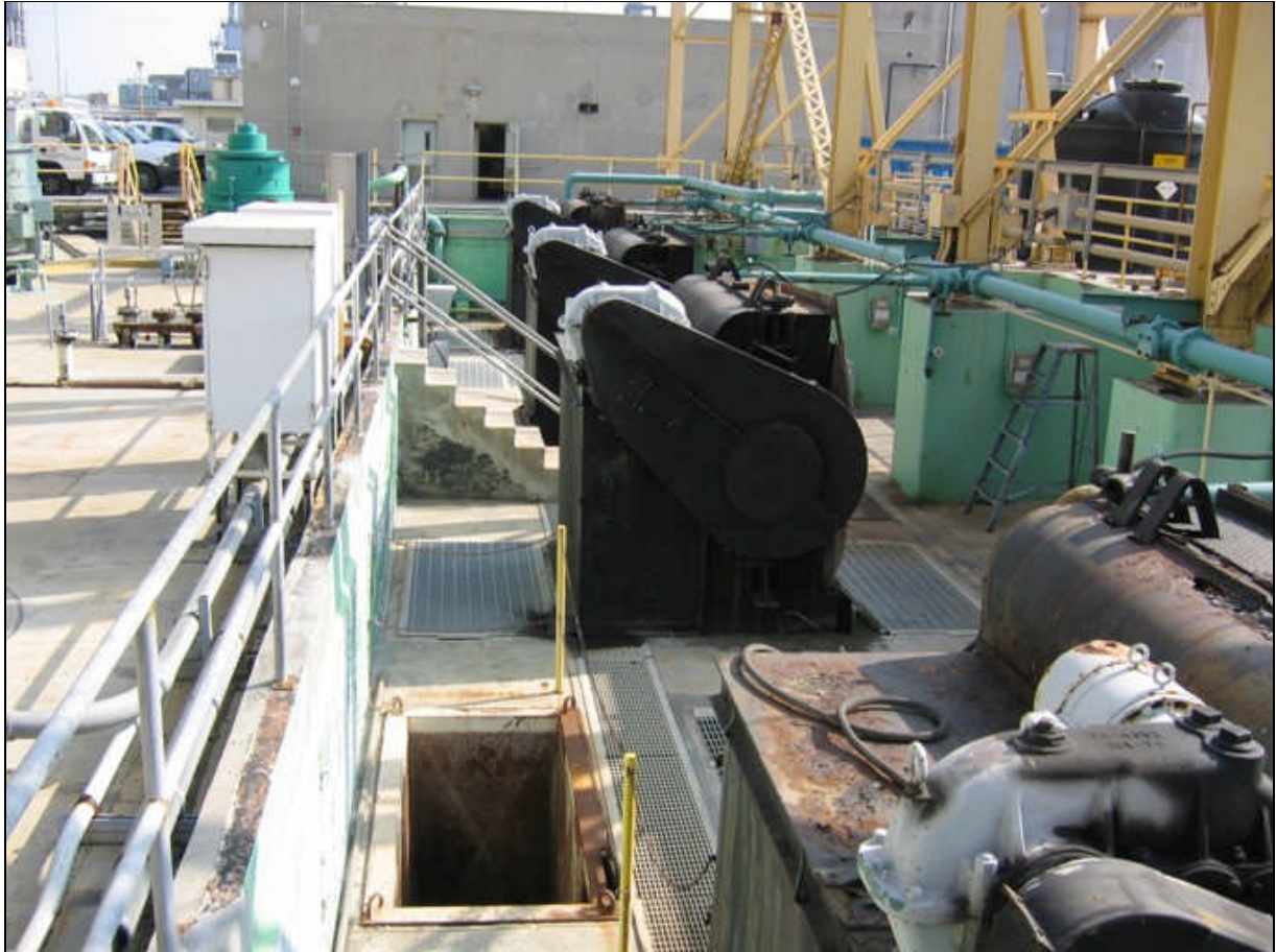
Figure A4-1. Unit 5 traveling screens.
