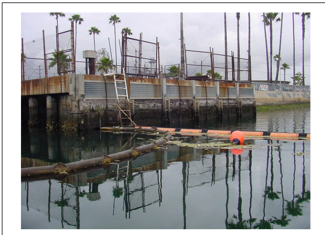
Figure 3.3-4. HGS intake structure near East Basin Channel in Inner Los Angeles Harbor.
