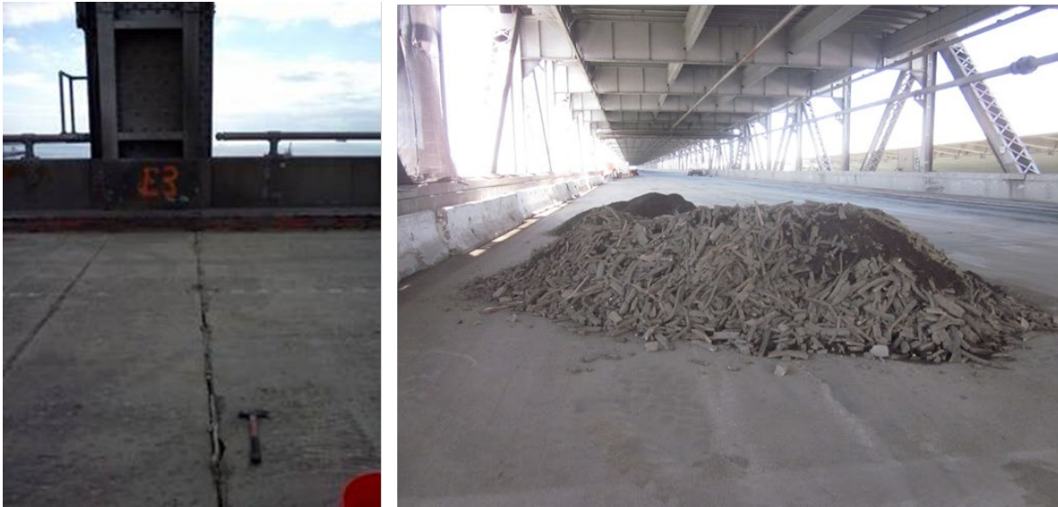
Figure 1-1. PCB-containing Caulk: PCB-containing caulk between road decks of the San Francisco Oakland Bay Bridge Old East span as discovered on inspection (left) and in a pile after removal (right), commingled with asphalt-concrete grindings.
