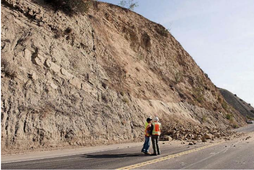
Figure C.26-1 Slopes Prone to Erosion and Sediment Discharge
