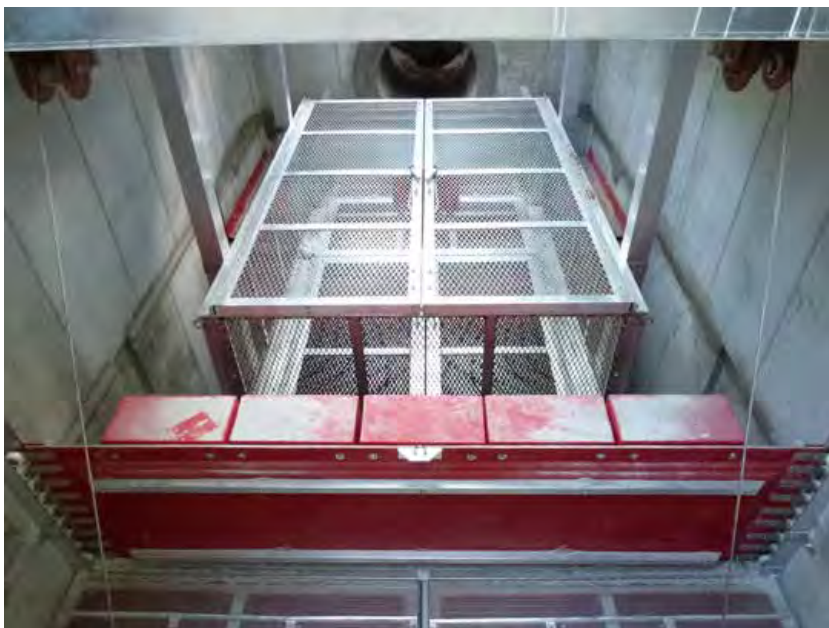
View of Nutrient Separating Baffle Box® and SkimBoss™ with Upflow Filter
