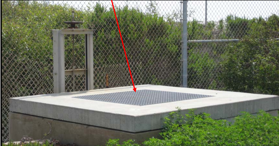
Figure 2.5.9 Stormwater collection point D14 South West Yard Drain south east of the insulator building.
