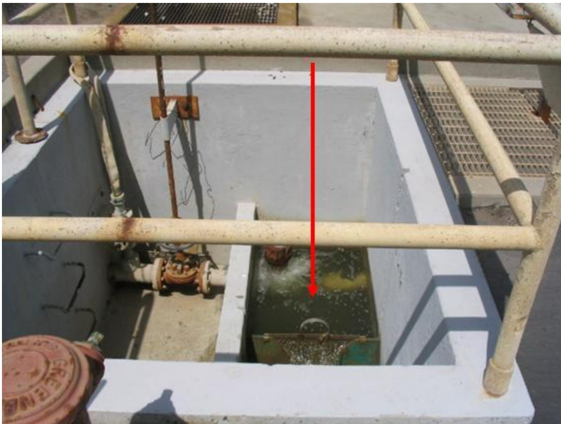
Figure 2.5.4. NPDES Low Volume Waste retention basins (water chemistry collection point).
