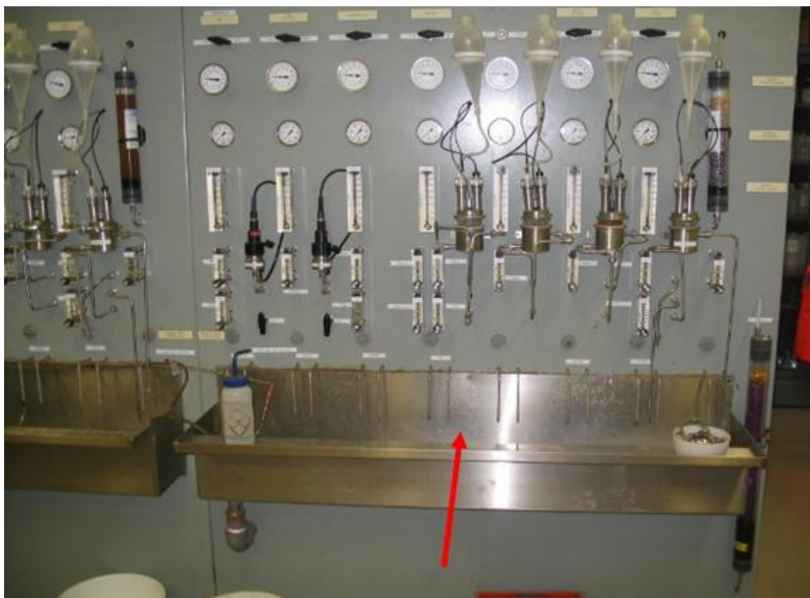
Figure 2.5.5. NPDES Low Volume Waste Boiler Blowdown Unit 1 (water chemistry collection point).
