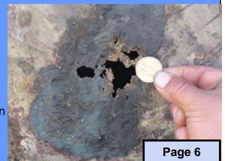
Photo 2: Hole in excavated UST
