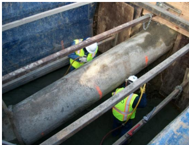
Pipelines transport water and add flexibility to water supply system operations.
