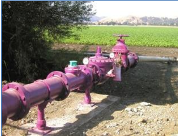
This pipeline in Gilroy provides recycled water to a local farmer
