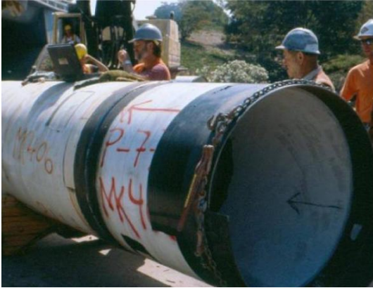
Pipelines and other infrastructure need periodic rehabilitation and replacement
