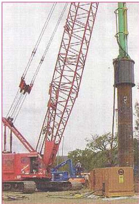
A Manitowoc 4000 crane and Lucas Marine's LMC 50 hydraulic impact hammer driving a 60-inch pile at Putah Creek.
