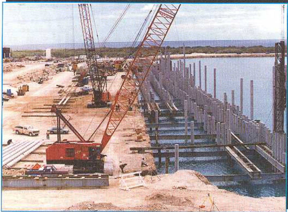
Hawaiian Dredging does its work at Barbers Point Harbor in Oahu, Hawaii.
