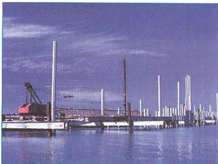
Hawaiian Dredging at work on Piers Five and Six at Barbers Point Harbor. More recently, the company did additional work at Pier Five and completed a project on Pier Seven.
