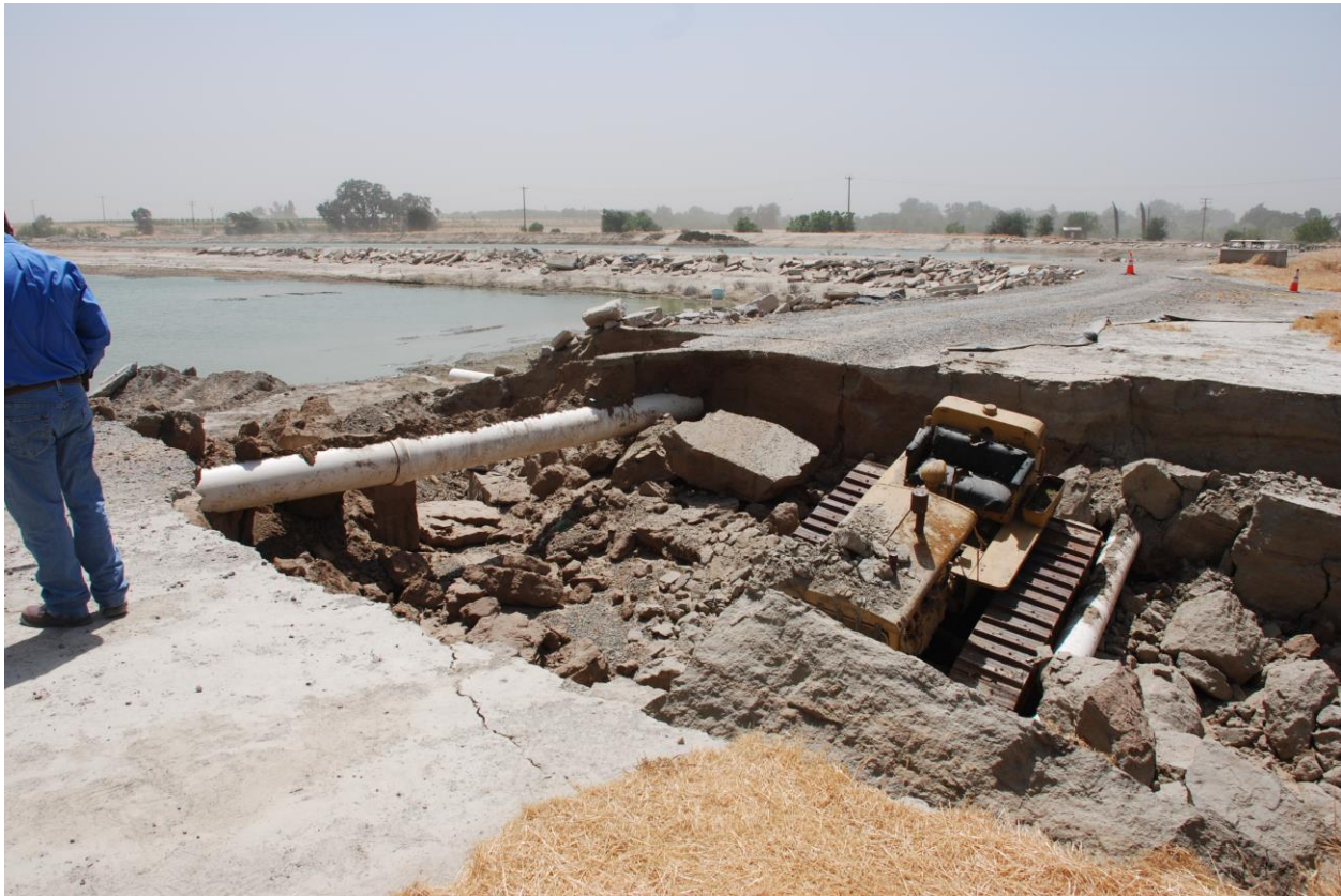
Caterpillar tractor in the broken Levee of wastewater holding basin.
