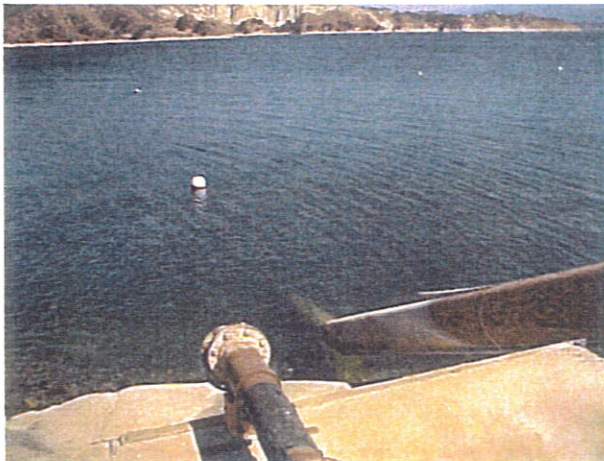
Water Intake Pipeline
