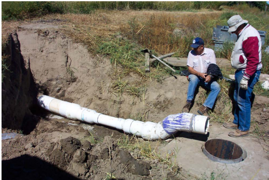
Figure 3. PID Ditch Rider Dennis Waggoner (l) and Ditch Superintendant Dan Korf (r) assisting with the May, 2003 pipe-fitting Venturi demonstration site installation
