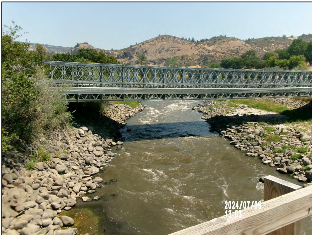
Figure D6b. Klamath River above Fall Creek near Copco, CA (USGS 11511990) - Daggett Bridge; upstream view. Taken July 9, 2024.
